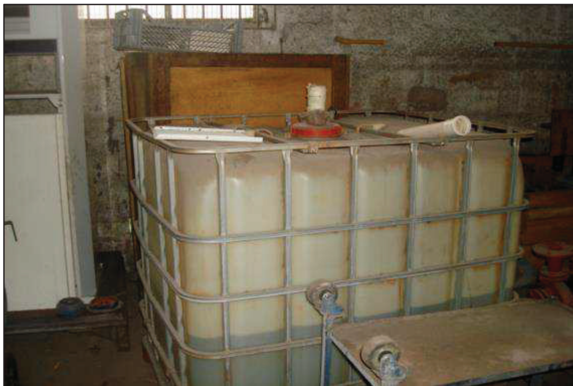
ITEM 5,345 - VISTA DO TANQUE GAIOLA 1000L
