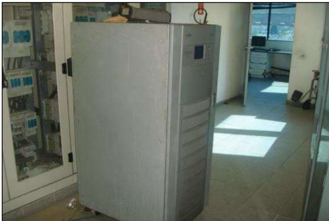
ITEM 1,800 - VISTA DO NOBREAK - EMERSON NETWORK POWER, 15KVA PN NXBOA0015C
