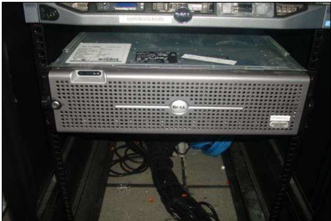
ITEM 1,353 - VISTA DO STORAGE DELL POWER VAULT MD3000I
