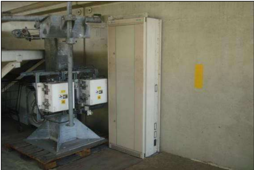
ITEM 1,822 - VISTA DO CENTRAL PABX ERICSSON MD 110
