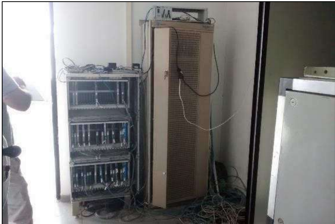
ITEM 1,411 - VISTA DO RACK MATEC MD 110 C 50 PLACAS
