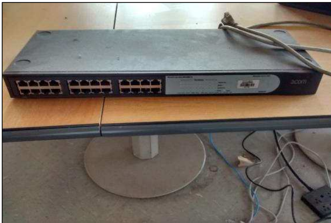
ITEM 1,331 - VISTA DO SWITCH 3COM 3C16471B
