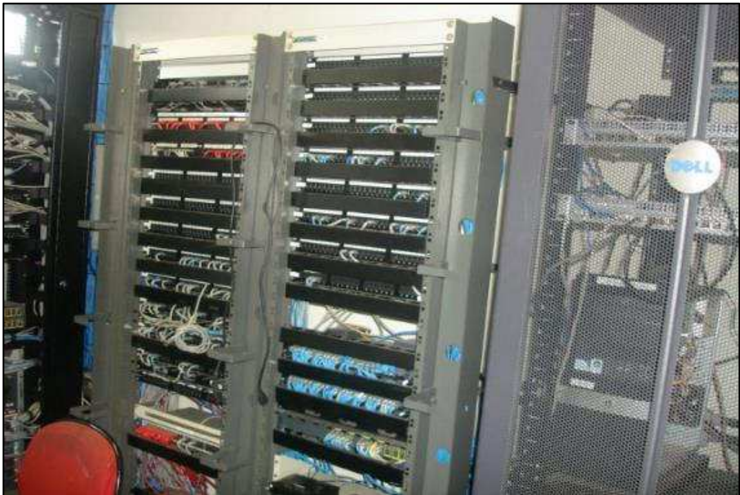
ITEM 1,340 - VISTA DO RACK DE TELECOM-
