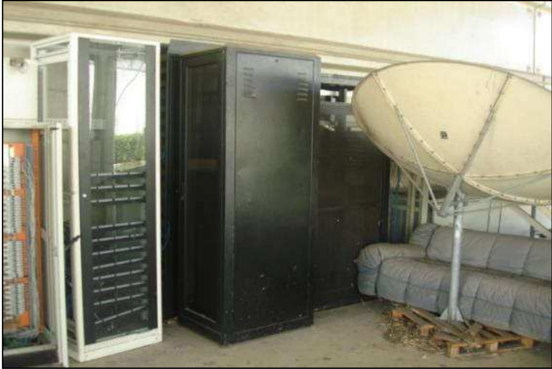
ITEM 1,817 - VISTA DO RACK SERVEROR
