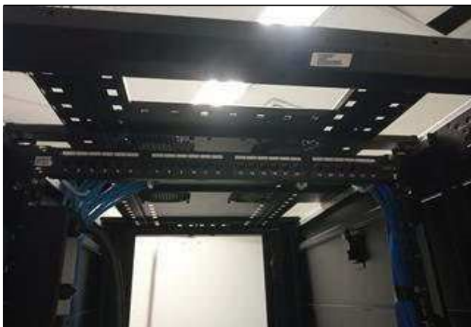
ITEM 1,403 - PATCH PANEL SOHO PLUS CAT6 LOCAL: SERVIDOR
