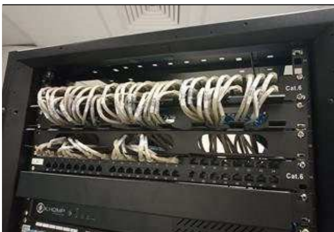
ITEM 1,405 - PATCH PANEL CAT6 LOCAL: SERVIDOR
