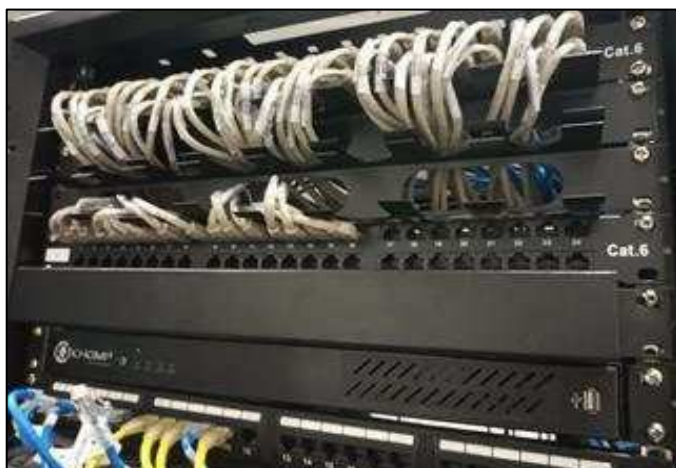
ITEM 1,406 - PATCH PANEL CAT6 LOCAL: SERVIDOR
