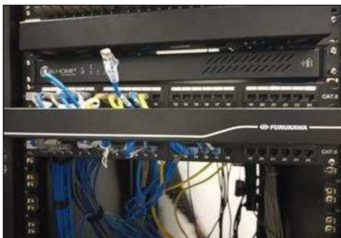
ITEM 1,408 - PATCH PANEL FURUKAWA CAT6 LOCAL: SERVIDOR
