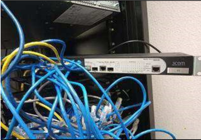
ITEM 1,421 - SWITCH 24 PORTAS 3COM BASELINE SWITCH 2226 SFP PLUS LOCAL: SERVIDOR
