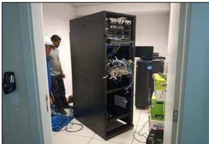
ITEM 1,404 - RACK SERVIDOR APC LOCAL: SERVIDOR
