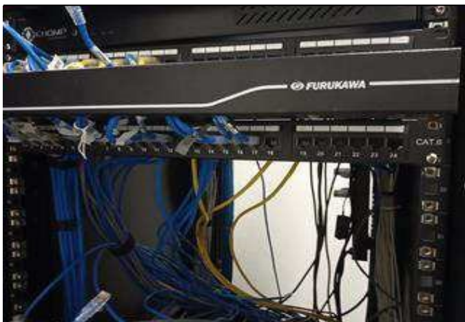
ITEM 1,409 - PATCH PANEL FURUKAWA CAT6 LOCAL: SERVIDOR
