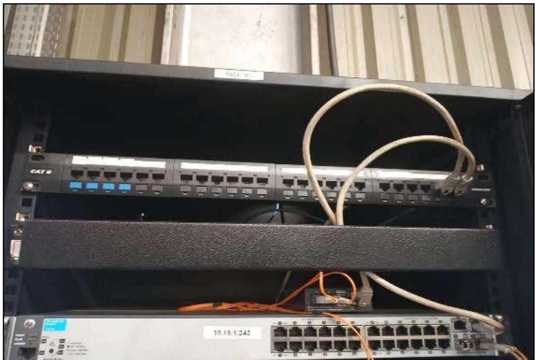
ITEM 3,002 - VISTA DO PATCH PANEL FURUKAWA CAT 6
