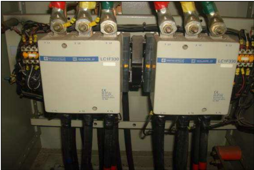
ITEM 1,877 - VISTA DO CONTATOR LC1 F330 TELEMECANIQUE
