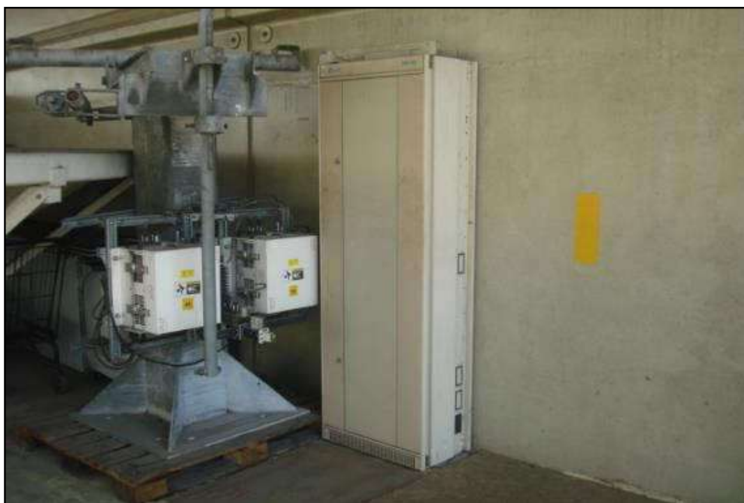
ITEM 1,822 - VISTA DO CENTRAL PABX ERICSSON MD 110
