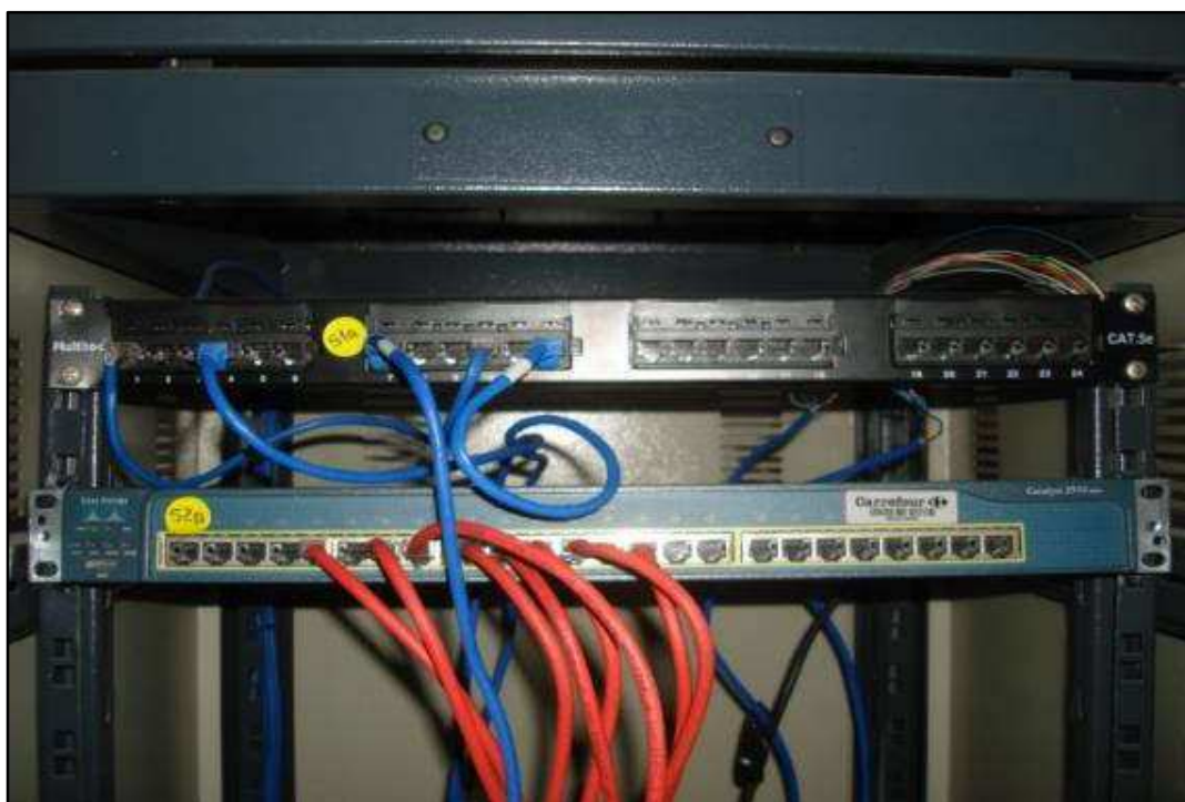
ITEM 0139 - VISTA DO SWITCH MARCA: CISCO SYSTEM MOD: CATALYST 2950
