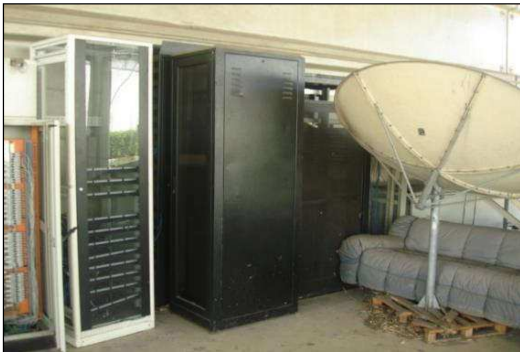
ITEM 1,817 - VISTA DO RACK SERVEROR
