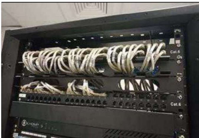
ITEM 1,405 - PATCH PANEL CAT6 LOCAL: SERVIDOR
