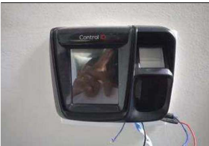
ITEM 1,389 - ACESSO BIOMÉTRICO CONTROL ID LOCAL: MARKETING
