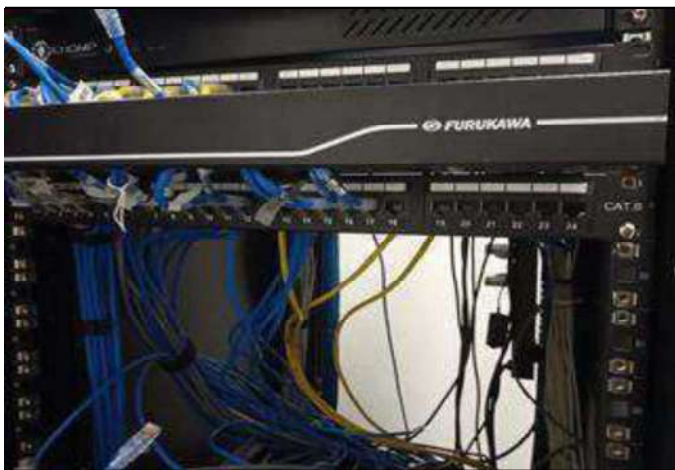
ITEM 1,409 - PATCH PANEL FURUKAWA CAT6 LOCAL: SERVIDOR
