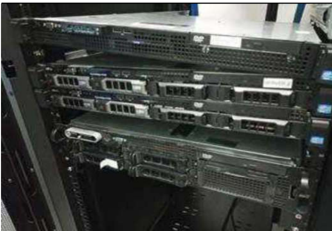
ITEM 1,401 - SERVIDOR DELL POWEREDGE R420 LOCAL: SERVIDOR
