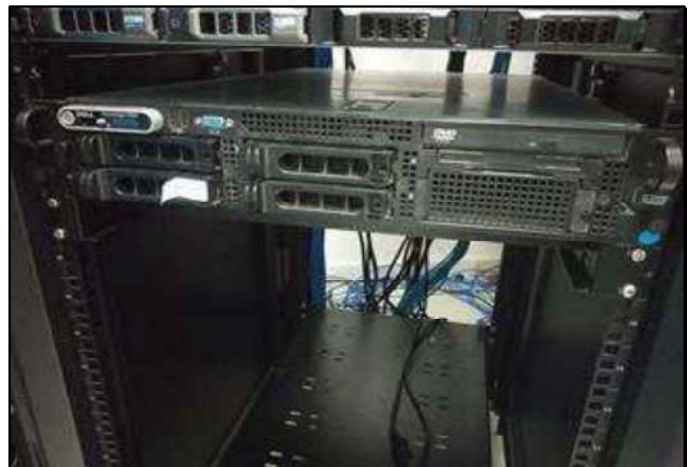
ITEM 1,402 - SERVIDOR DELL POWEREDGE 2950 LOCAL: SERVIDOR
