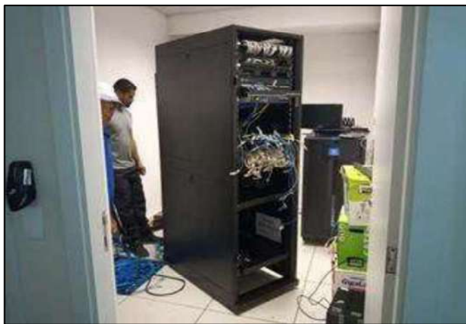
ITEM 1,404 - RACK SERVIDOR APC LOCAL: SERVIDOR
