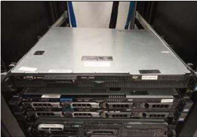
ITEM 1,399 - SERVIDOR DELL POWEREDGE R210 II LOCAL: SERVIDOR
