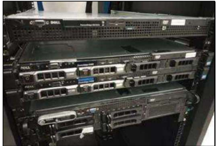
ITEM 1,400 - SERVIDOR DELL POWEREDGE R420 LOCAL: SERVIDOR
