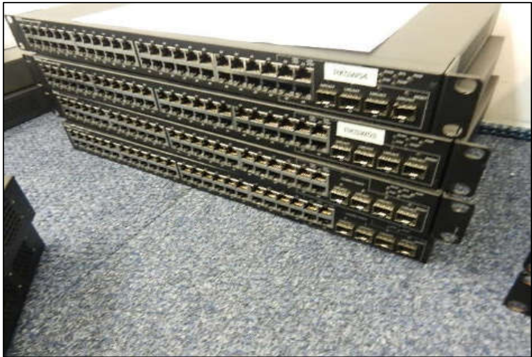
ITEM 0095 - SWITCH DELL POWERCONNECT 5448
