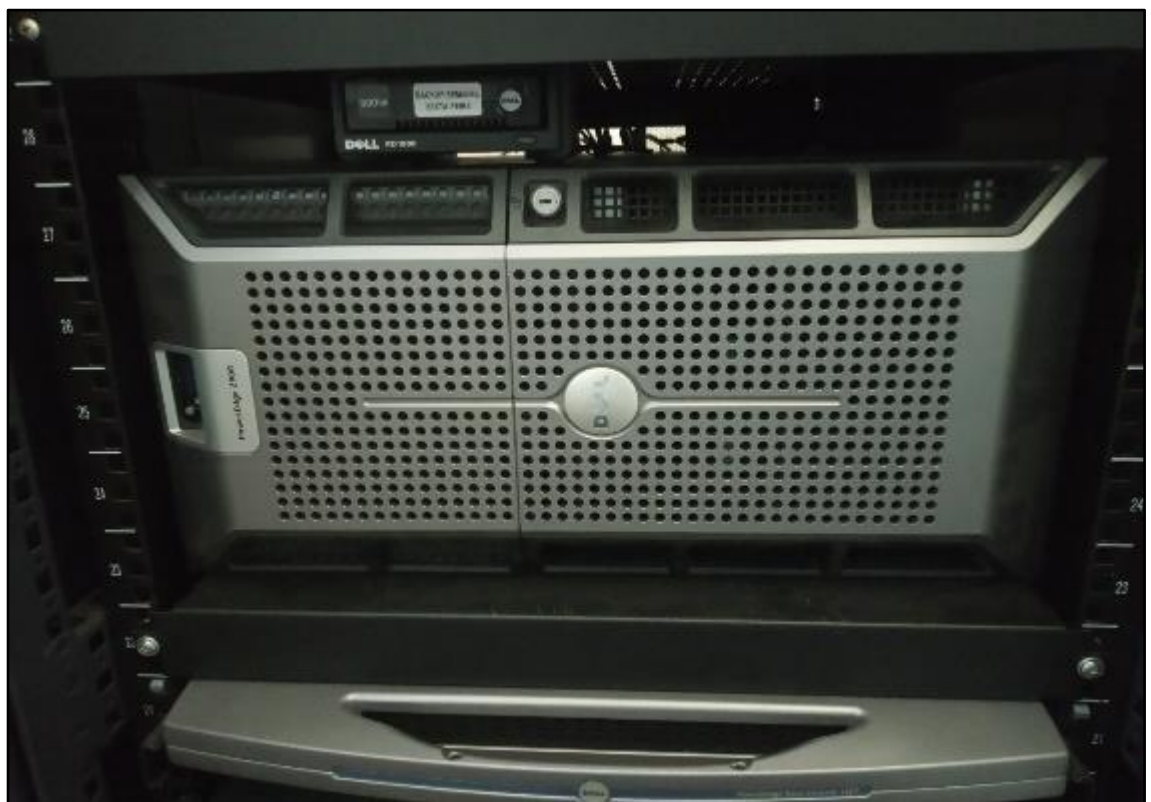
ITEM 3,056 - VISTA DO SERVIDOR DELL POWEREDGE 2900
