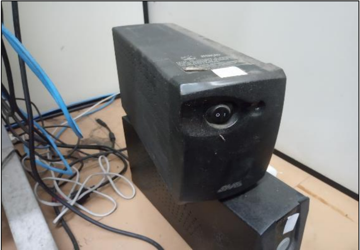
ITEM 3,128 - VISTA DO NOBREAK SMS NETSTATION ST600SFX
