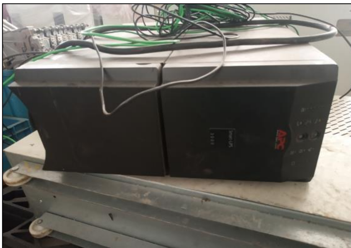
ITEM 3,130 - VISTA DO NOBREAK APC SMART UPS 3000
