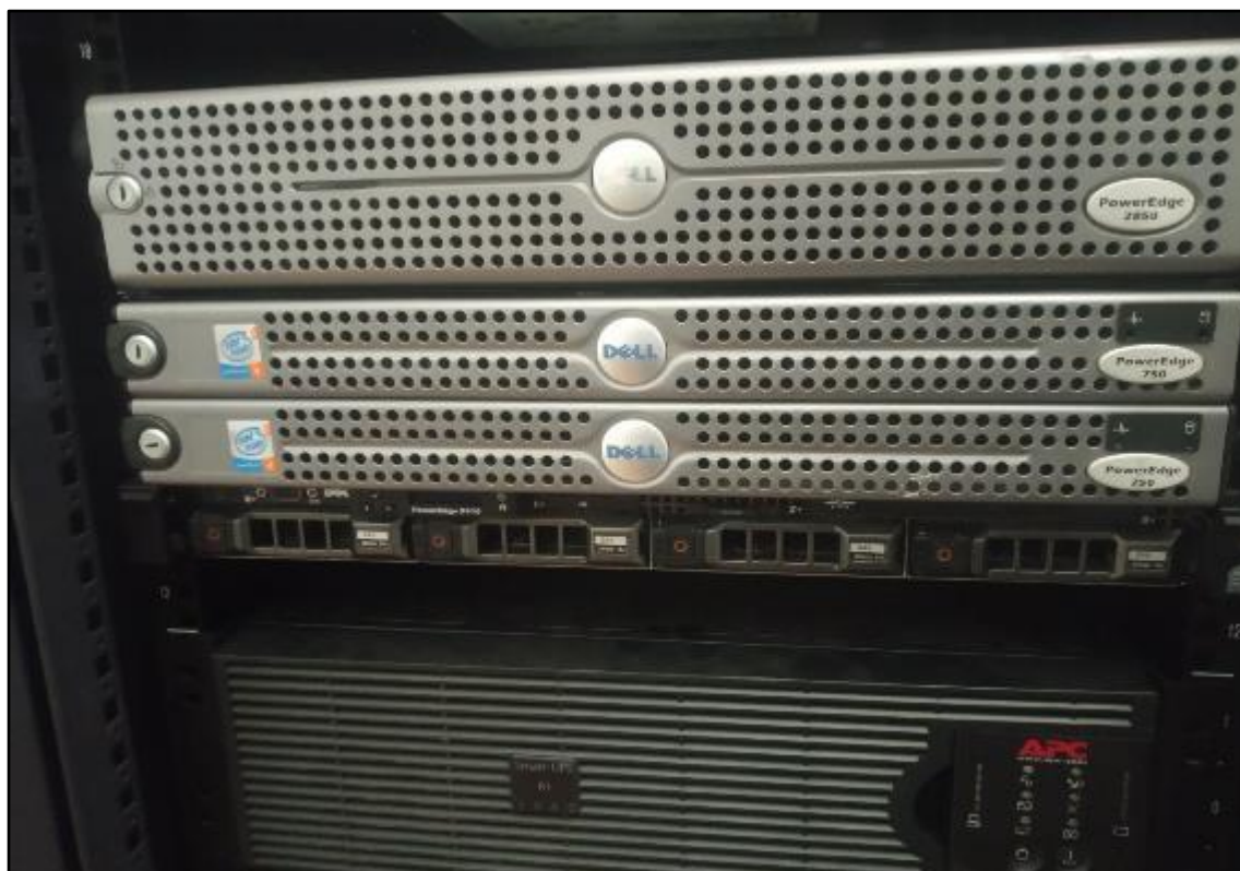
ITEM 3,059 - VISTA DO SERVIDOR DELL POWEREDGE 750
