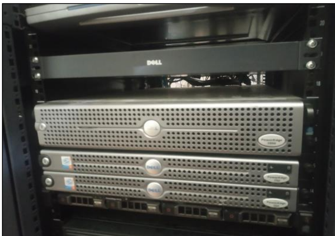
ITEM 3,058 - VISTA DO SERVIDOR DELL POWEREDGE 2850
