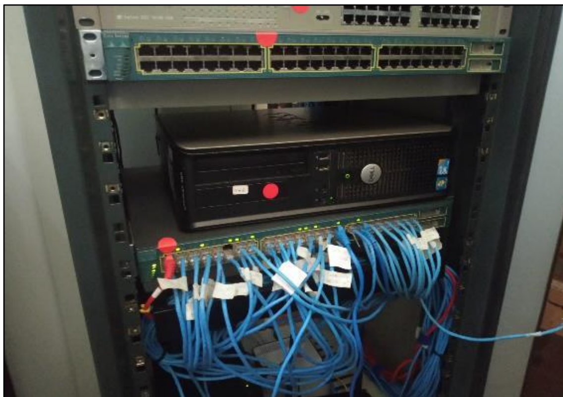
ITEM 3,047 - VISTA DO SWITCH CISCO CATALYST 3550
