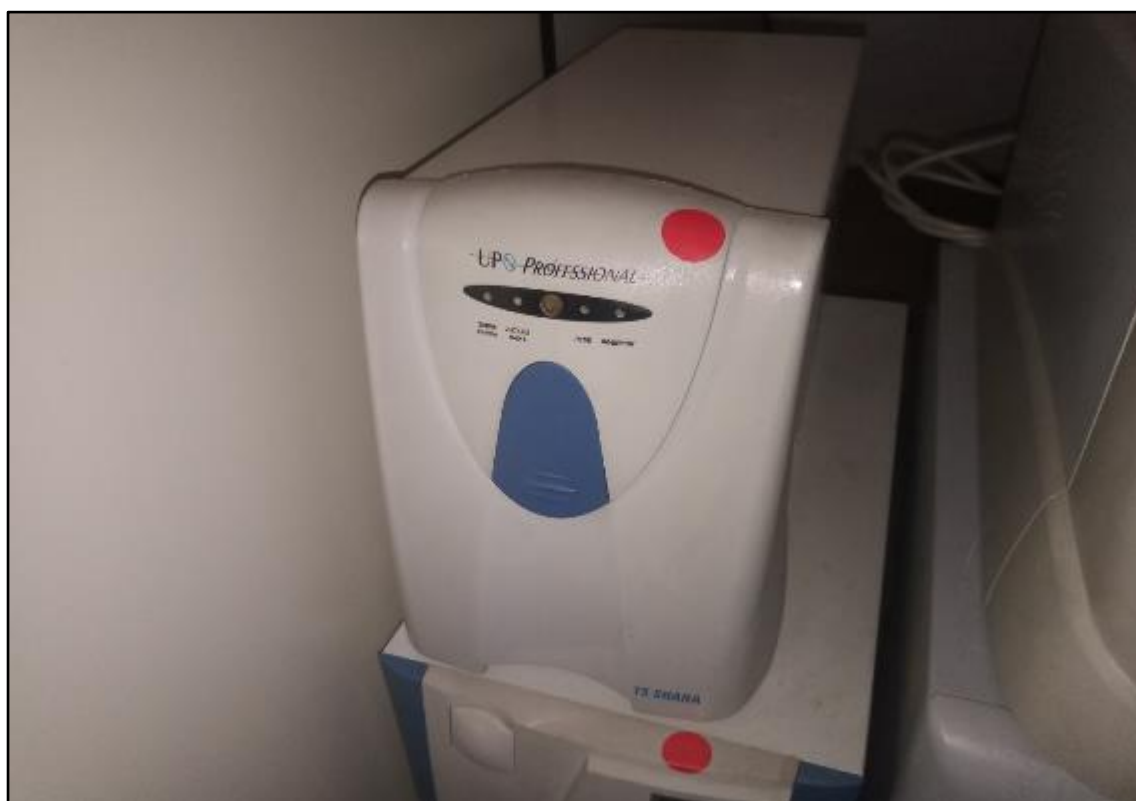
ITEM 3,017 - VISTA DO NOBREAK TS SHARA UPS 1600
