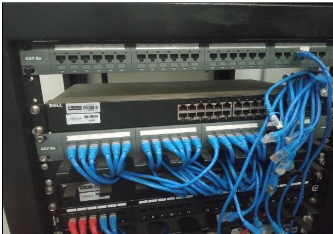
ITEM 3,038 - VISTA DO PATCH PANEL FURUKAWA CAT5E
