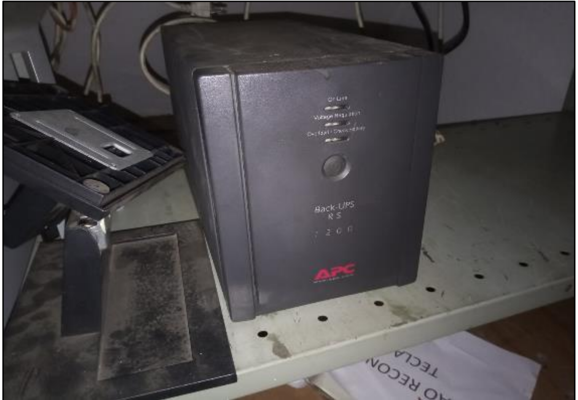
ITEM 3,013 - VISTA DO NOBREAK APC BACK UPS RS 1200
