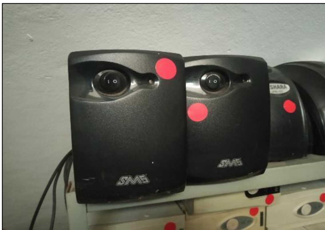
ITEM 3,006 - VISTA DO NOBREAK SMS NETSTATION
