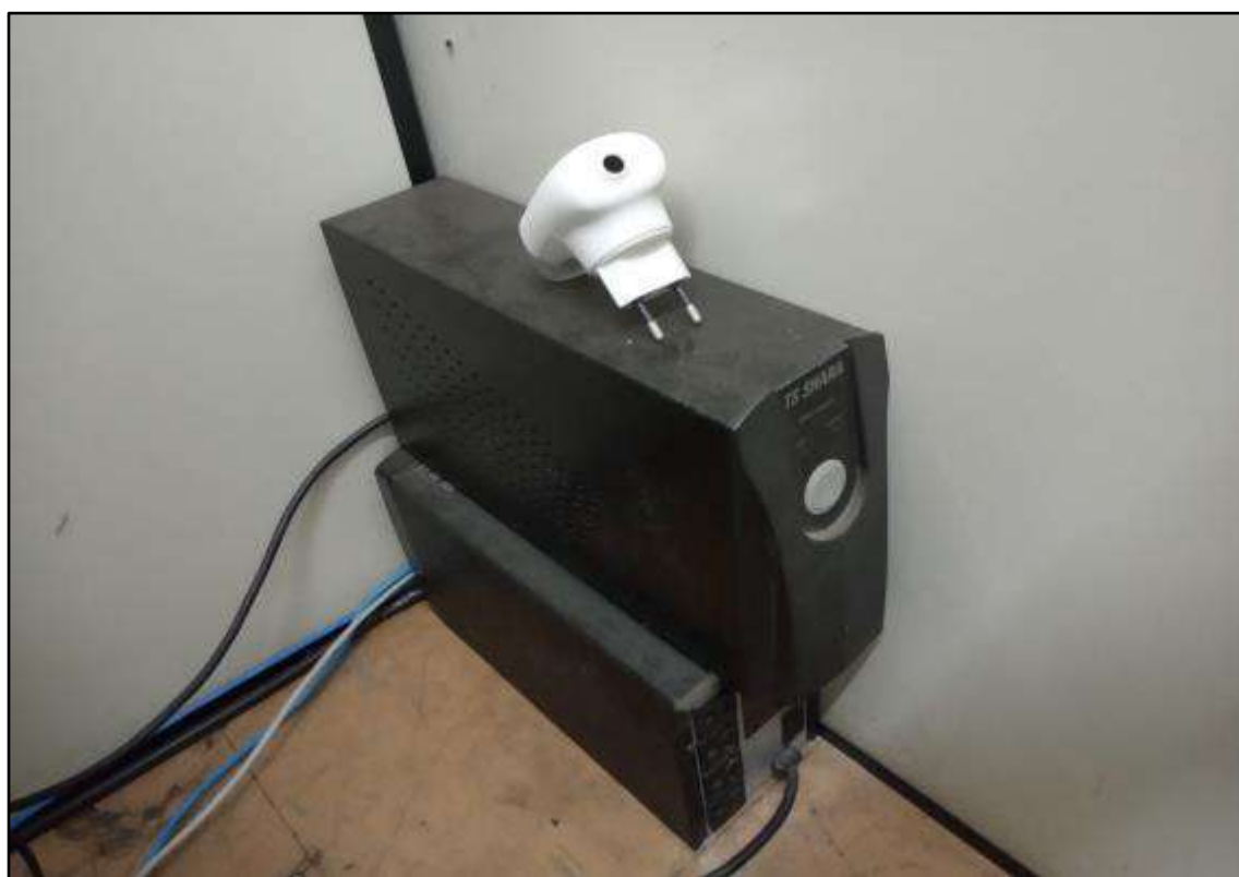
ITEM 3,127 - VISTA DO NOBREAK TS SHARA UPS COMPACT 600
