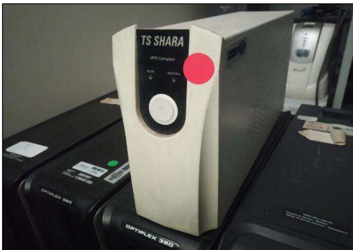
ITEM 3,010 - VISTA DO NOBREAK TS SHARA UPS COMPACT 600
