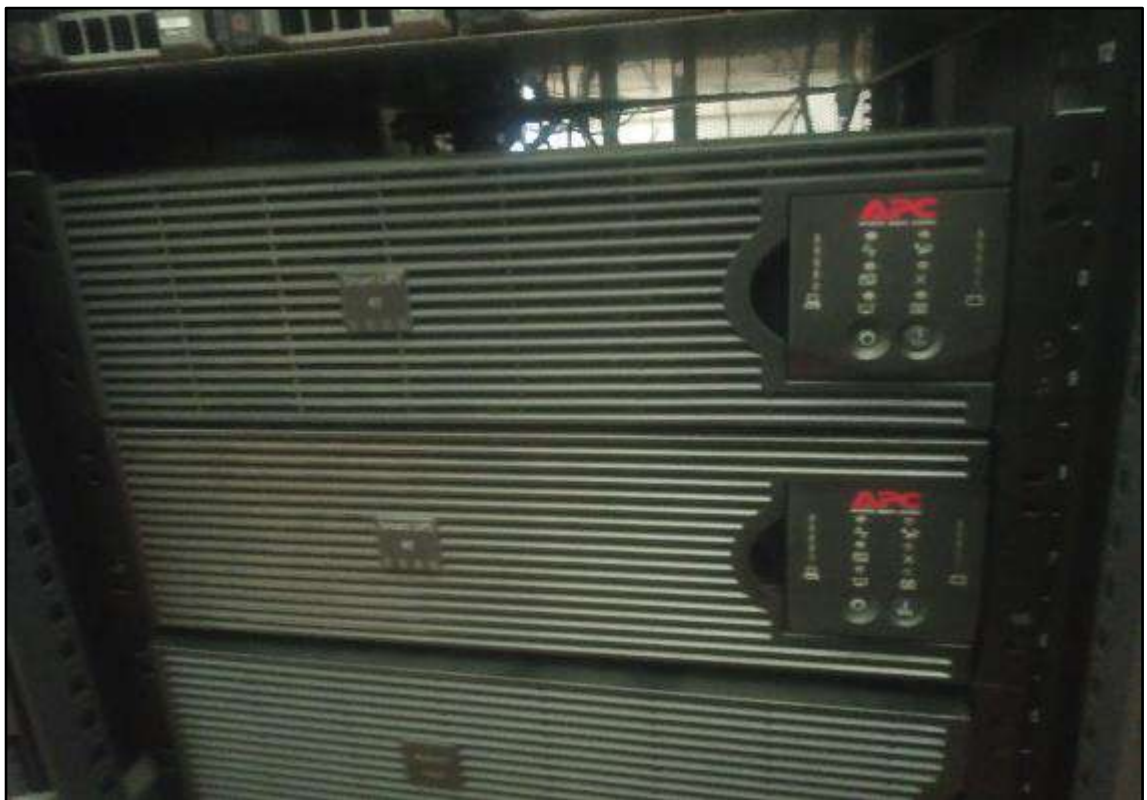
ITEM 3,061 - VISTA DO NOBREAK APC SMART UPS RT 5000
