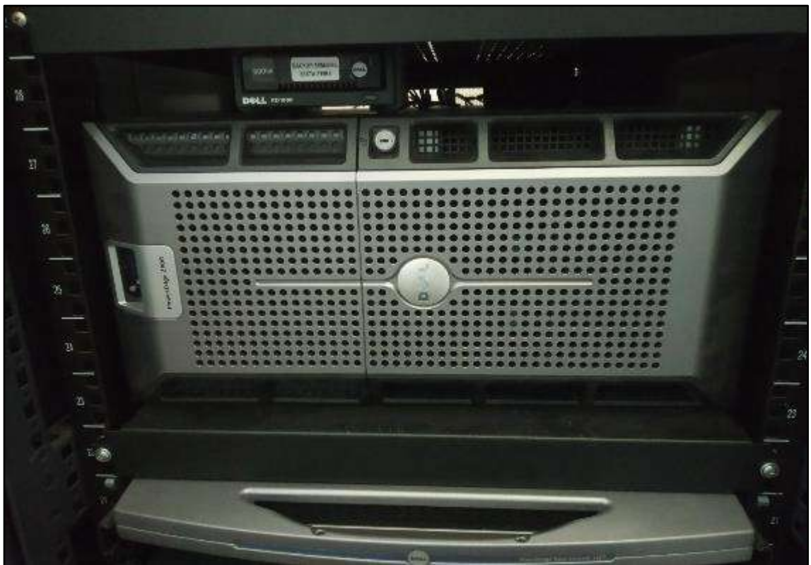
ITEM 3,056 - VISTA DO SERVIDOR DELL POWEREDGE 2900
