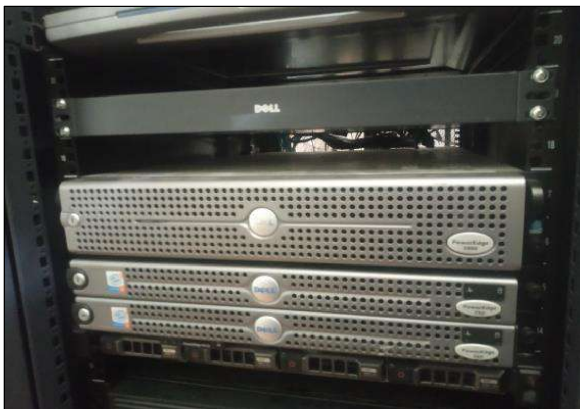
ITEM 3,058 - VISTA DO SERVIDOR DELL POWEREDGE 2850
