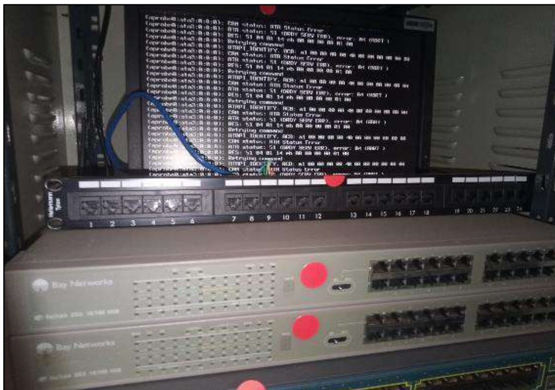
ITEM 3,045 - VISTA DO PATCH PANEL HELLEMAN TYTON
