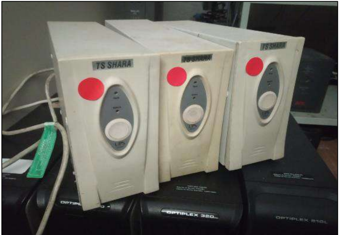
ITEM 3,008 - VISTA DO NOBREAK TS SHARA UPS COMPACT 500 PLUS
