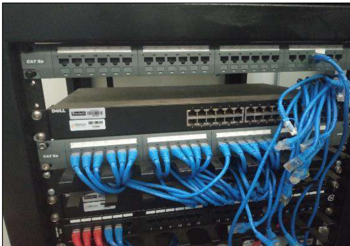
ITEM 3,038 - VISTA DO PATCH PANEL FURUKAWA CAT5E
