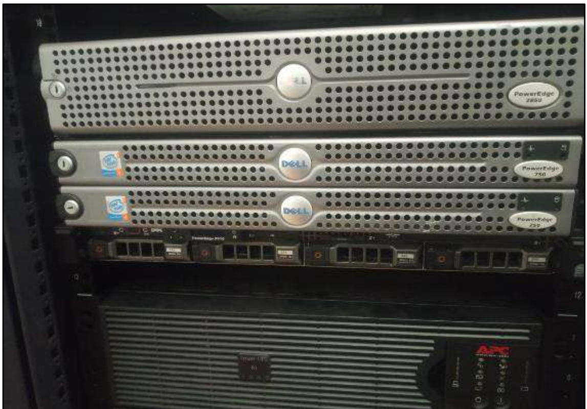
ITEM 3,059 - VISTA DO SERVIDOR DELL POWEREDGE 750
