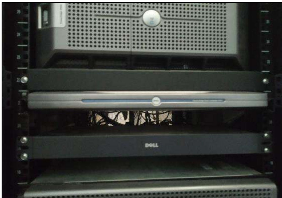
ITEM 3,057 - VISTA DO CONSOLE DELL POWEREDGE RACK CONSOLE 15FP
