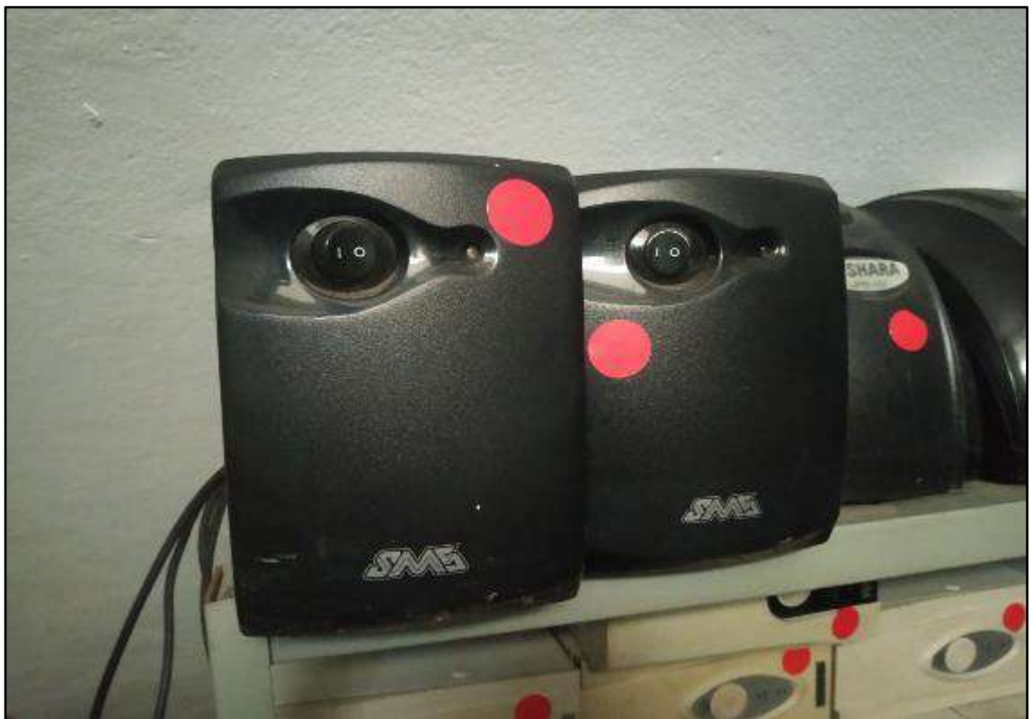
ITEM 3,006 - VISTA DO NOBREAK SMS NETSTATION
