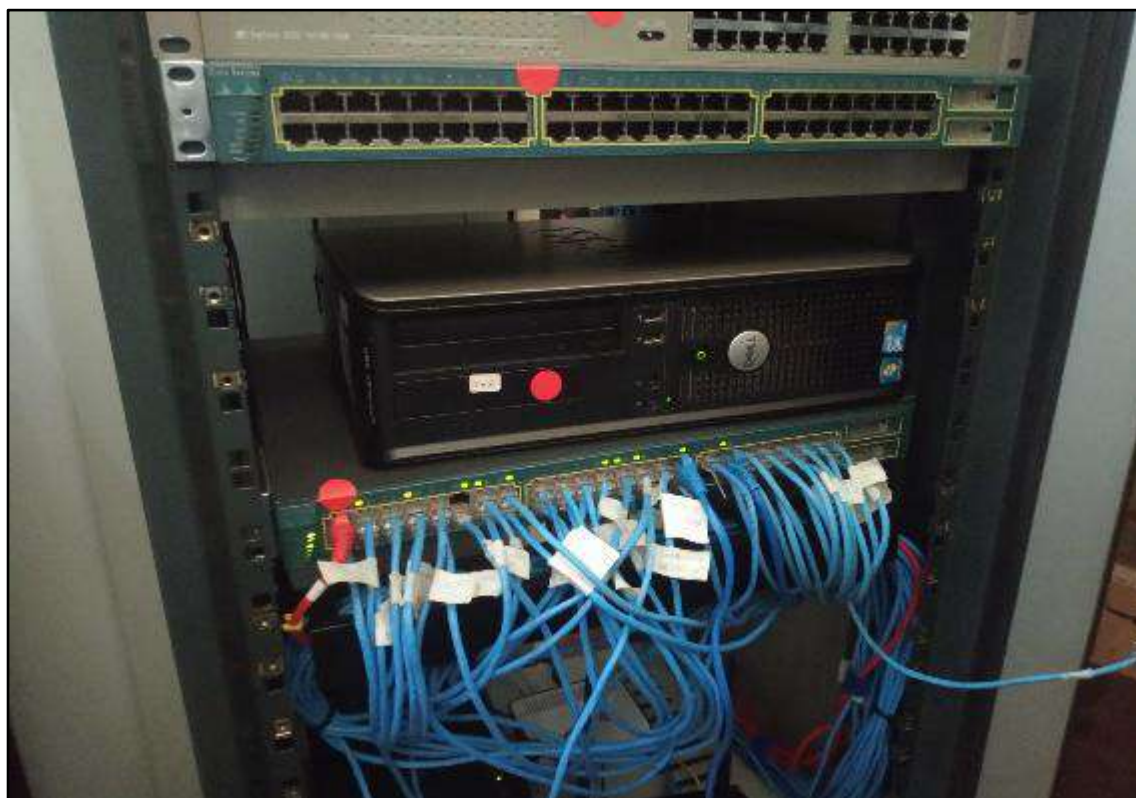
ITEM 3,047 - VISTA DO SWITCH CISCO CATALYST 3550
