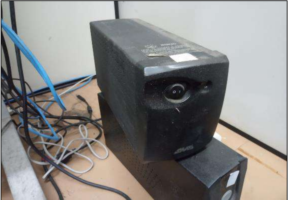
ITEM 3,128 - VISTA DO NOBREAK SMS NETSTATION ST600SFX
