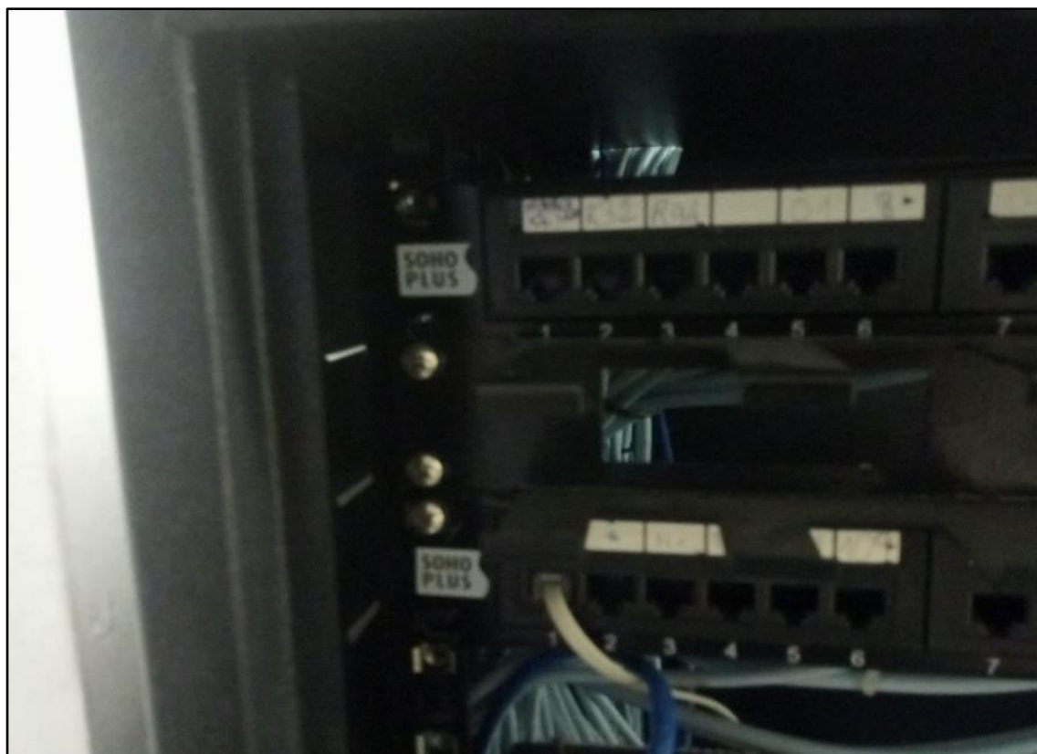
ITEM 2,018 - RACK SUSPENSO COM 6 PATCH PANEL
