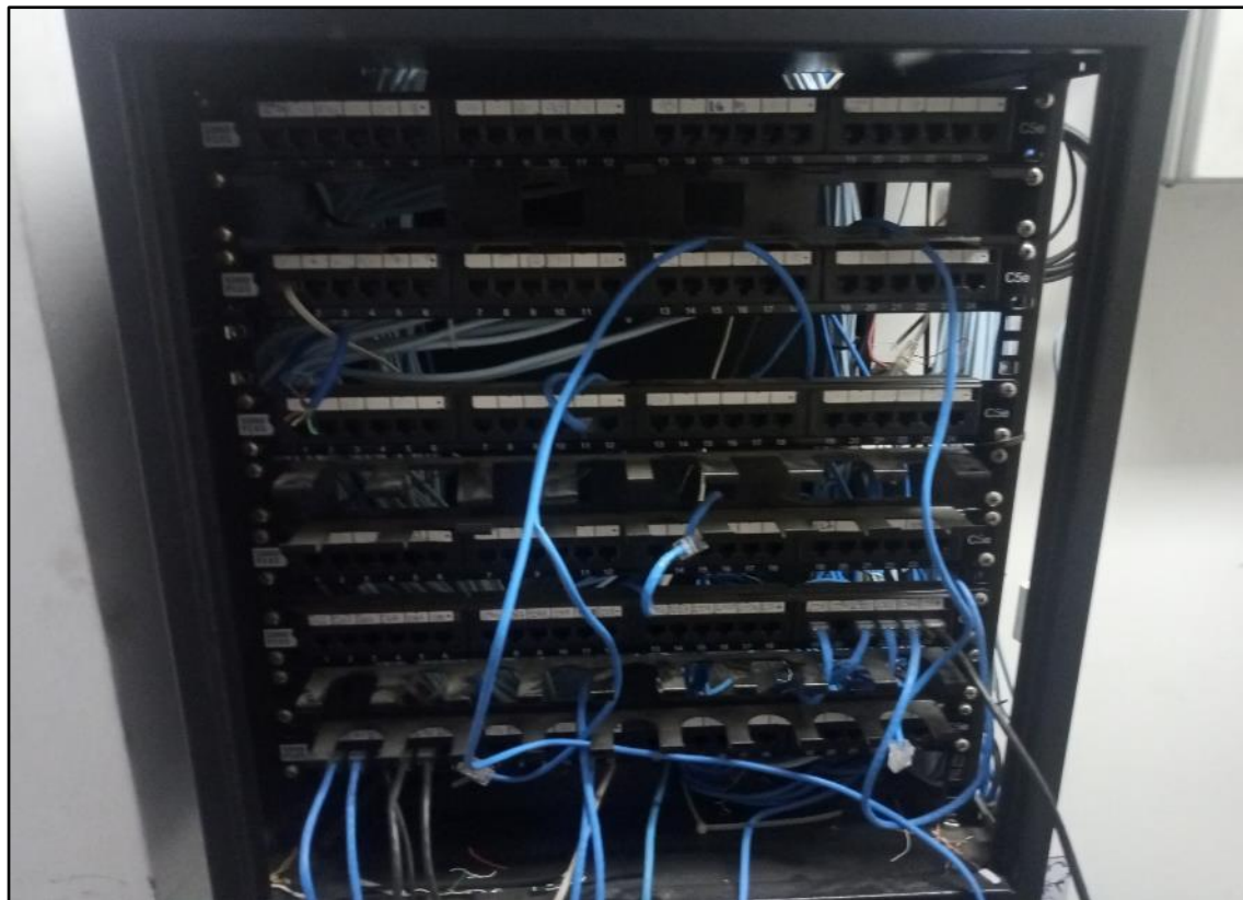
ITEM 2,018 - RACK SUSPENSO COM 6 PATCH PANEL
