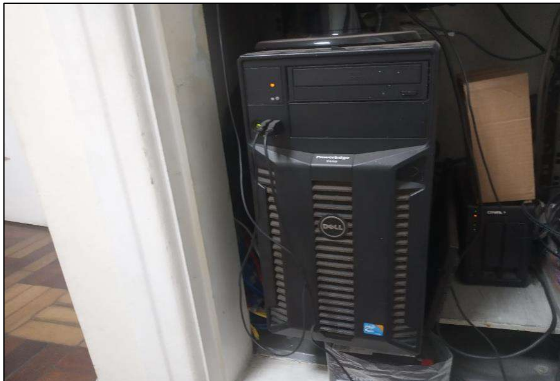
ITEM 3,020 - VISTA DO SERVIDOR DELL POWEREDGE T410 SERVICE TAG JLKZ8S1
