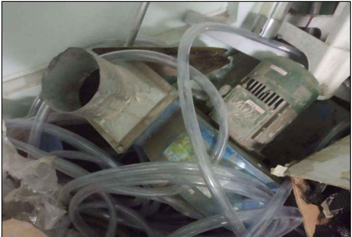
ITEM 1,026 - VISTA DO EXAUSTOR INDUSTRIAL
