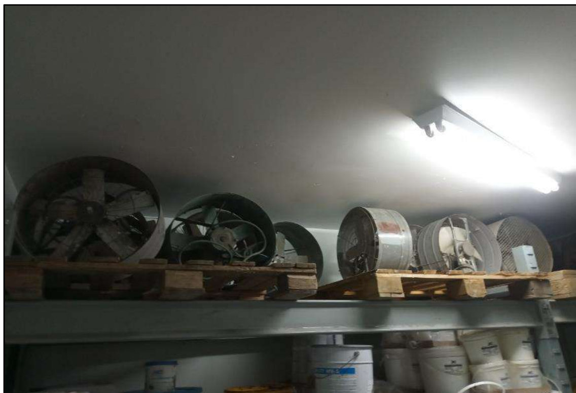
ITEM 1,002 - VISTA DO EXAUSTOR
