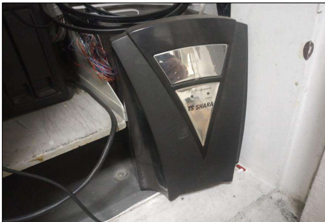
ITEM 3,024 - VISTA DO NO BREAK TS SHARA UPS PROFESSIONAL 1200
