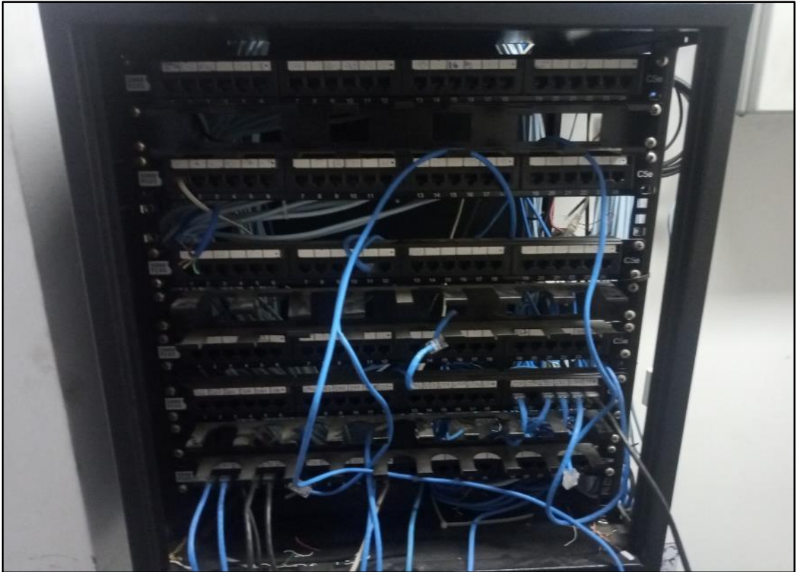
ITEM 2,018 - RACK SUSPENSO COM 6 PATCH PANEL
