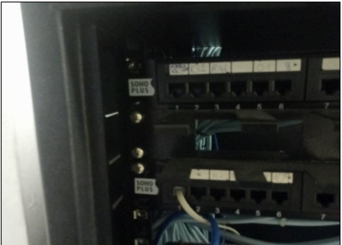
ITEM 2,018 - RACK SUSPENSO COM 6 PATCH PANEL
