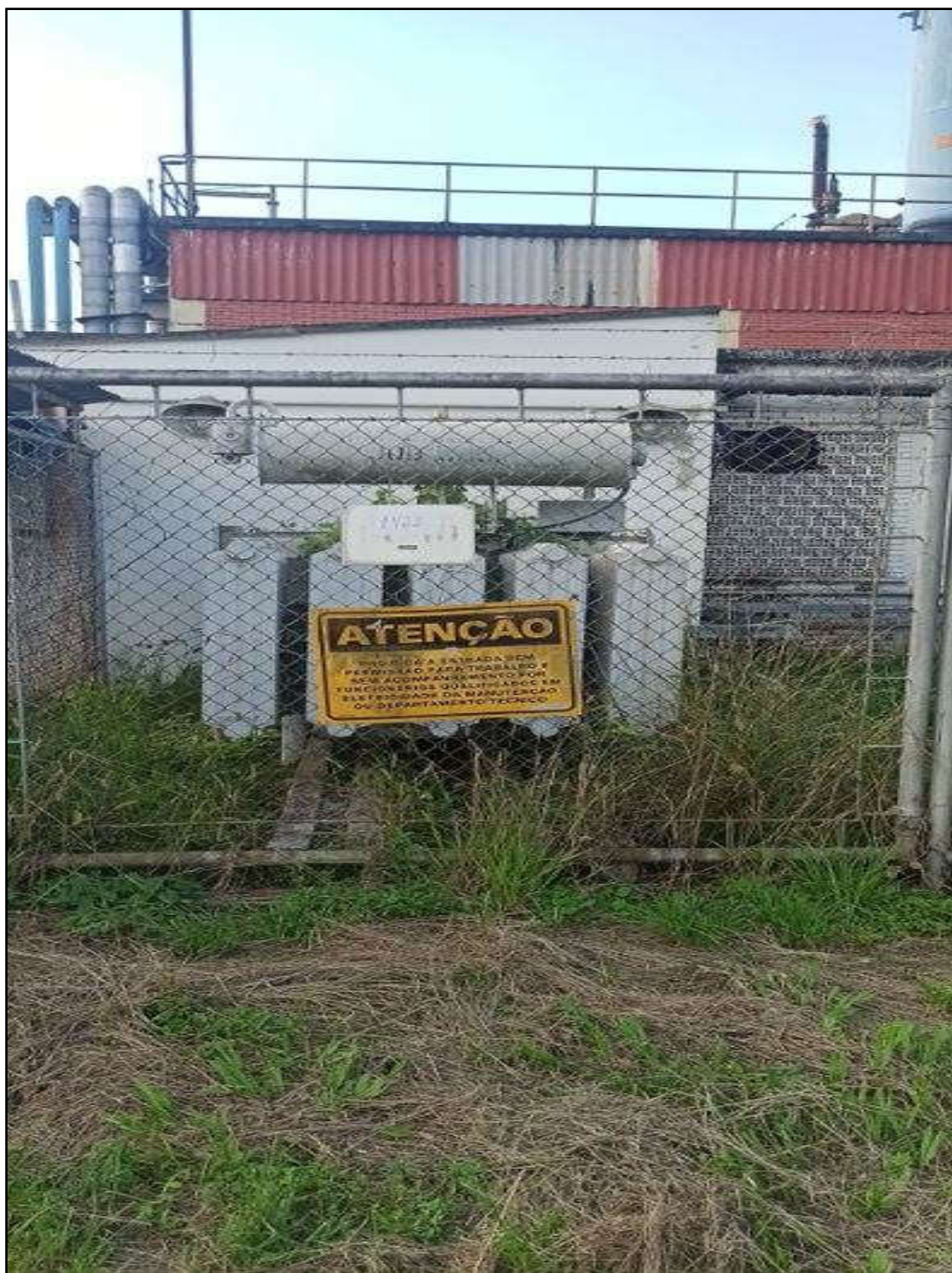
ITEM 1,004 – VISTA DO TRANSFORMADOR TRIFASICO A OLEO, FAB. DEDINI, MOD. T3-1000-15/1.2.LF.LF.C, TENSAO ENT./SAIDA 13,8 KV/480 V, POT. 1,0 MVA
