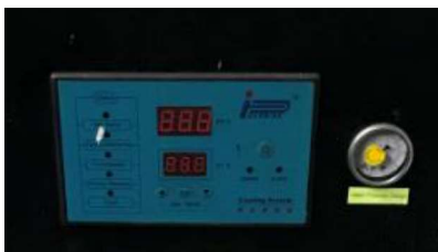
(Fig 03 – Painel de comando principal)
