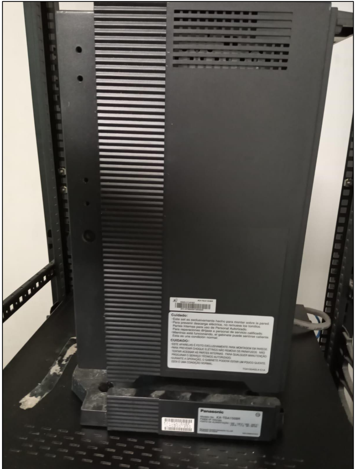
ITEM 2,007 - CENTRAL PABX PANASONIC KX-TDA1508
