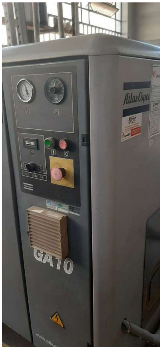
COMPRESSOR ATLAS COPCO GA10
