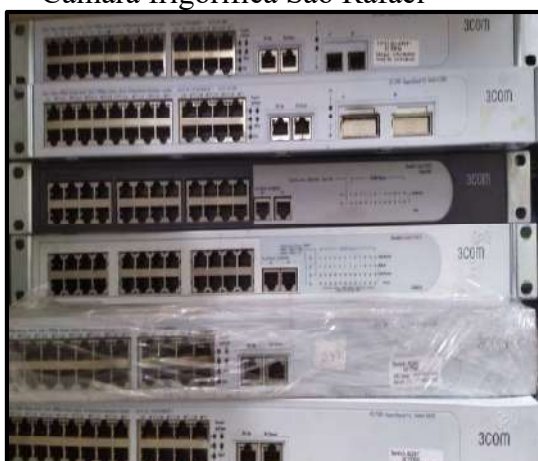
Switches 24 portas 3COM
