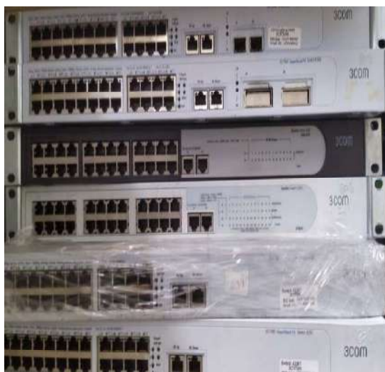
Switches 24 portas 3COM
