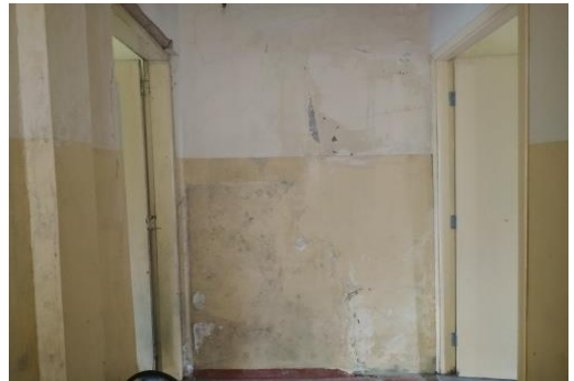
Hall parede infiltrada
